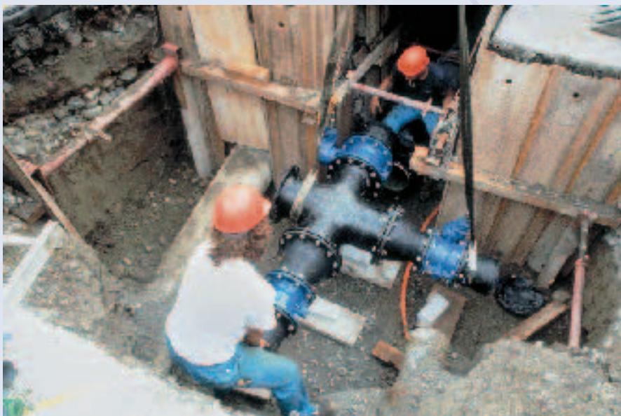
Municipal Water Supply Zurich
