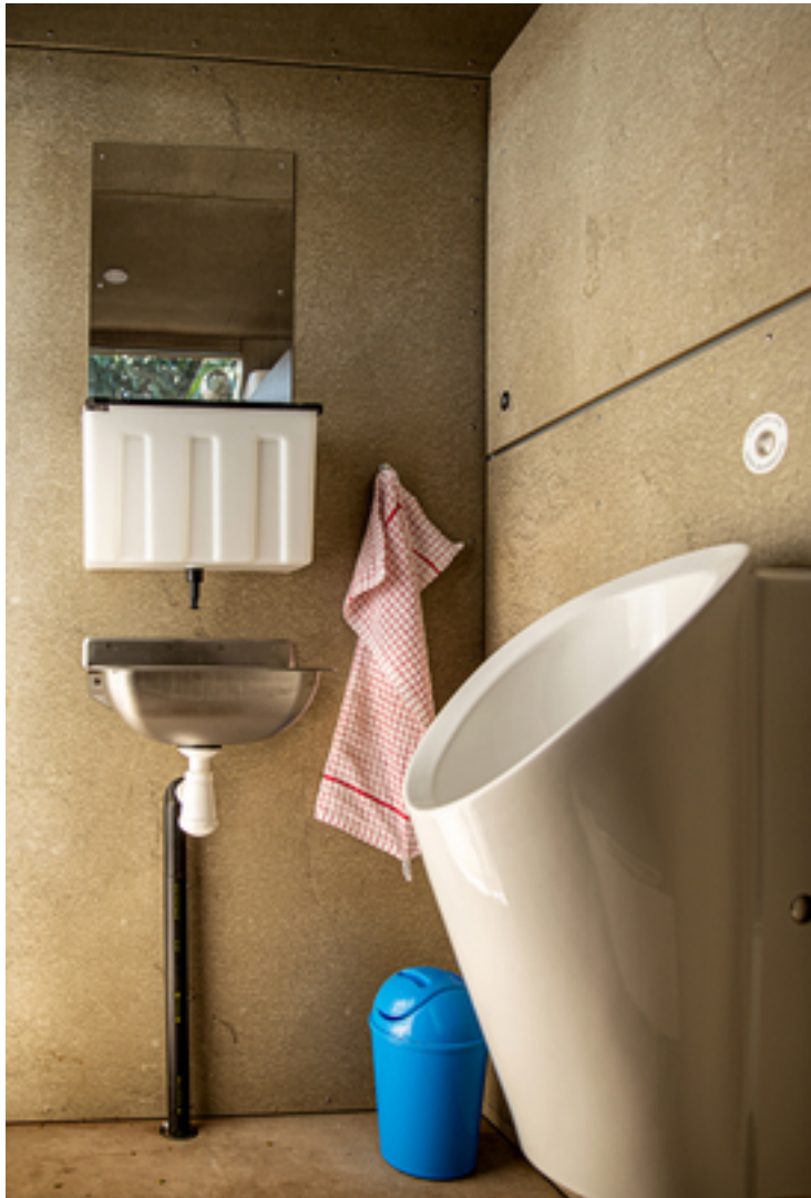
Urinal and wash basin in the Blue Diversion Autarky toilet cubicle in Durban. The separation toilet is not shown. Photo: Autarky, Eawag
