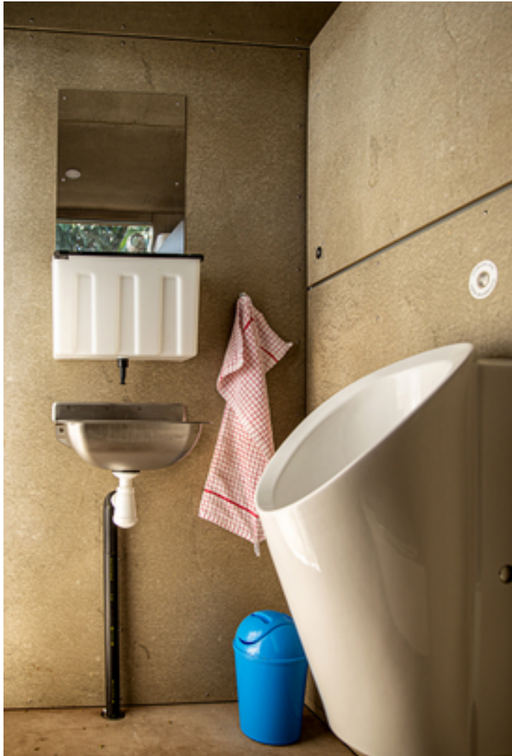
Urinal and wash basin in the Blue Diversion Autarky toilet cubicle in Durban. The separation toilet is not shown. Photo: Autarky, Eawag
