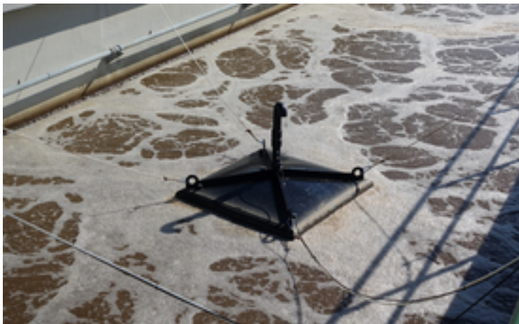
Off-gas measurement hood in operation at the Birs WTP. (Photo: Andrin Moosmann)
