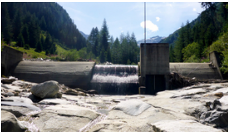
The weir of the Wannebode small hydroelectric power station near Reckingen (VS) interrupts the continuum of the Blinnenbach. (Photo: Eawag)
