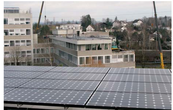
The solar panel on the roof of Forum Chriesbach. A photovoltaic system is also to be installed on the roof of the old office building (back) when the refurbishment and upper storey addition is complete.
