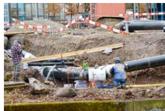
On the Eawag/Empa site, construction workers laid new pipes for the mid-temperature network.
