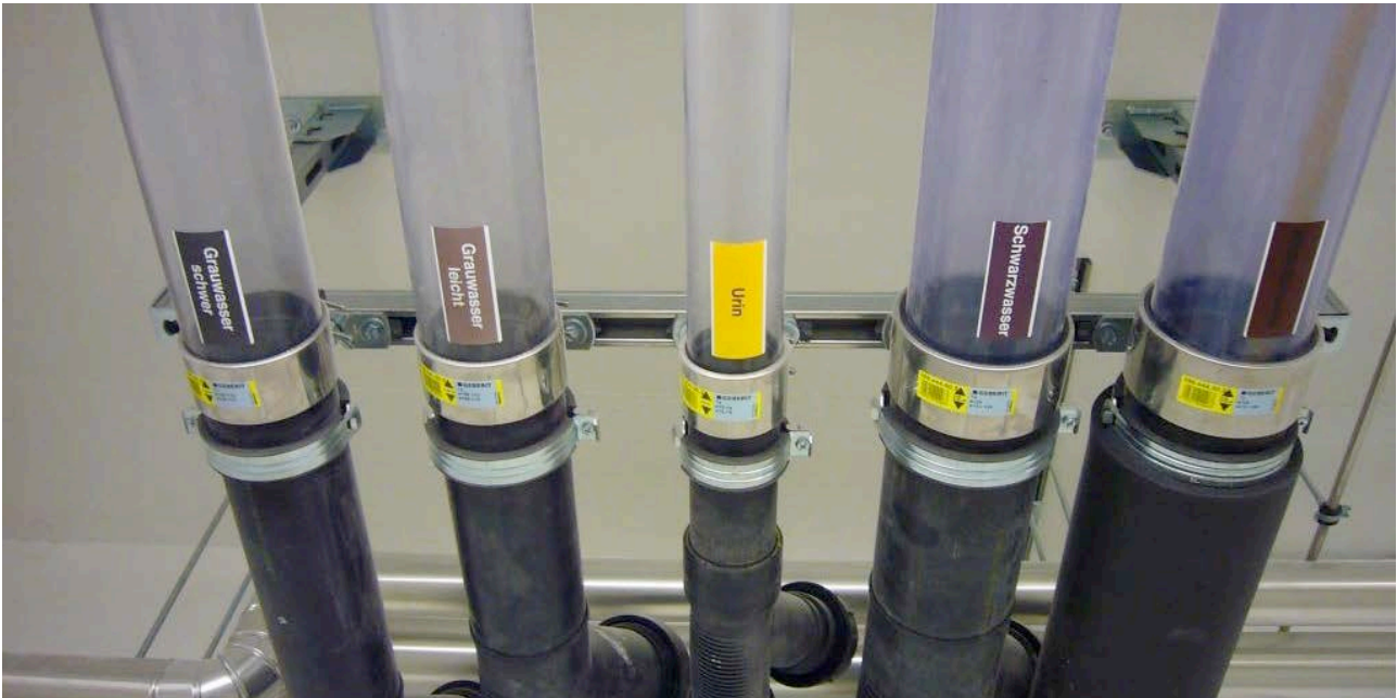
Figure 1. Five different pipes convey the various wastewater types to the Water Hub: light and heavy greywater, urine, brownwater, and mixed wastewater. Not on the picture: rainwater pipe.
