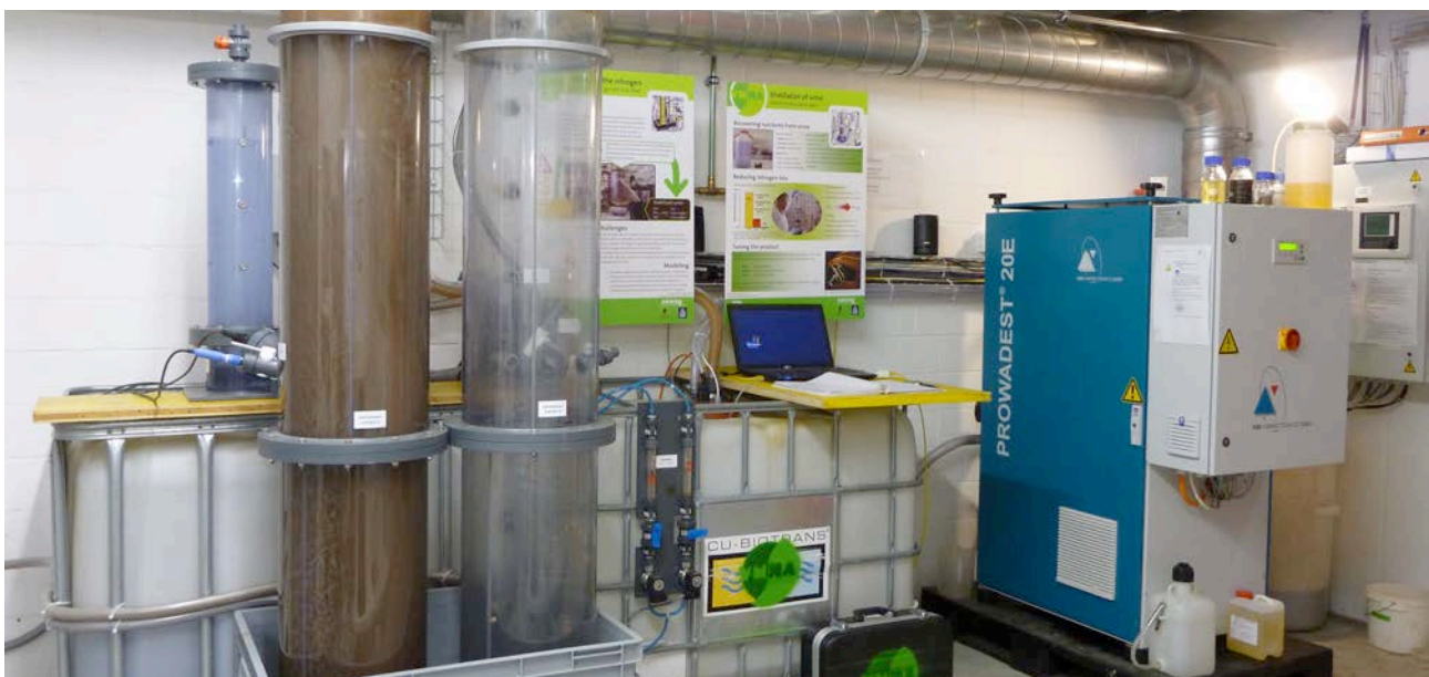
Figure 3. The VUNA moving-bed biofilm reactor stabilises the urine, before it is concentrated in an industrial distiller to produce a liquid fertiliser. A similar reactor is installed in the Water Hub.
