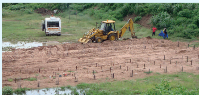
Figure 5.4 The Umlazi Deep Row Entrenchment Test Site – top the burial of faecal sludge from pit latrines in 1 m deep trenches; below an overview picture of the filled trenches with trees planted on top. Groundwater wells were mapped to follow the fate of nutrients, organics and pathogens (photos: Jay Bhagwan, Water Research Council, South Africa).
