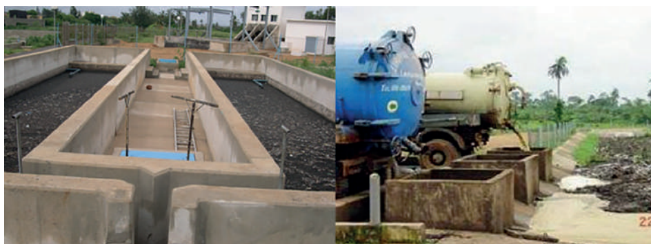
Figure 6.2 Left: the twin settling-thickening tanks of Rufisque faecal sludge management plant, in Dakar, Senegal. The operating cycle lasts two weeks (one week loading, one week desludging), and sludge is transferred to drying beds with a pump. Right: the settling-thickening pond in Achimota, Accra, Ghana, has an operational cycle of 8 weeks (4 weeks loading, 4 weeks desludging). As the sludge is thickened for four times as long, it is not possible to remove it with a pump, and manual extraction is carried out (photo: SANDEC).
