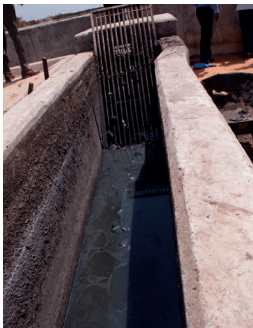
Figure 8.5 A holding -mixing tank with a bar screen is used in Senegal to prevent garbage from clogging the bed (photo: Linda Strande).
