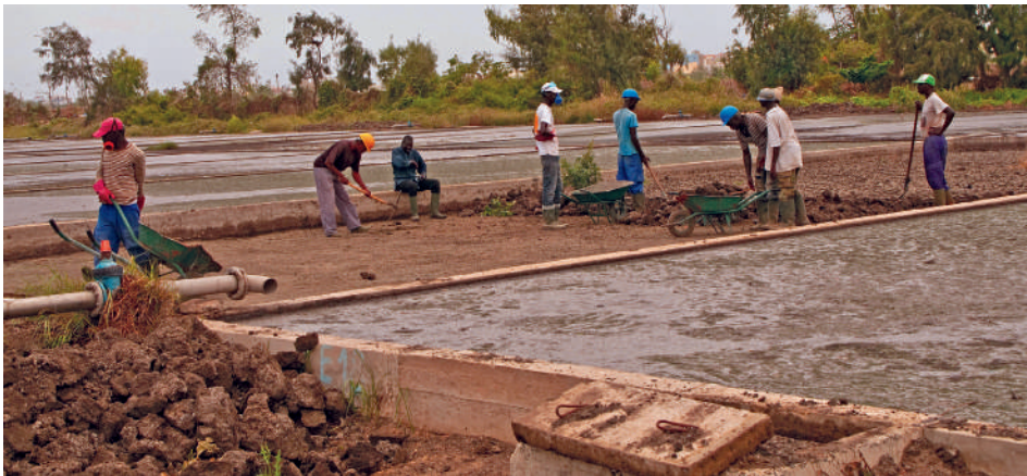
Figure 12.2 Harvesting of sludge from drying bed for use in agriculture, Dakar, Senegal (photo: Linda Strande).
