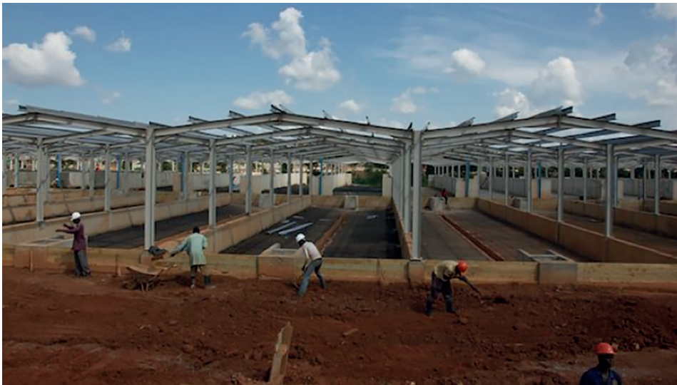
Figure 18.1 Drying beds for faecal sludge treatment under construction at Lubigi faecal sludge treatment plant in Kampala as part of the Lake Victoria Protection Stage I Project funded by KfW, EU and Government of Uganda/NWSC (photo: Lars Schoebitz).
