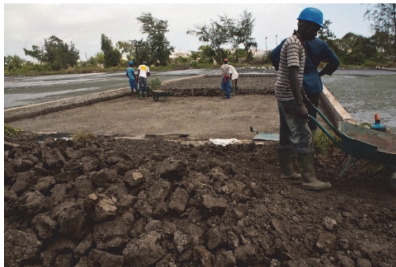
Figure 2.10 Removal of semi-solid to solid dewatered sludge from drying beds at Camberene treatment plant in Dakar, Senegal (photo: Eawag).
