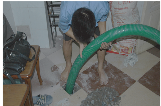
Figure 3.13 A septic tank located below a house, requiring the floor to be broken for emptying or sampling, Hanoi, Vietnam (photo: Eawag).
