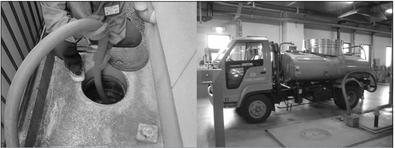
Fig. 5. Mobile sludge removal vehicle (reprinted with permission from Matsui et al. 27 © IWA)
