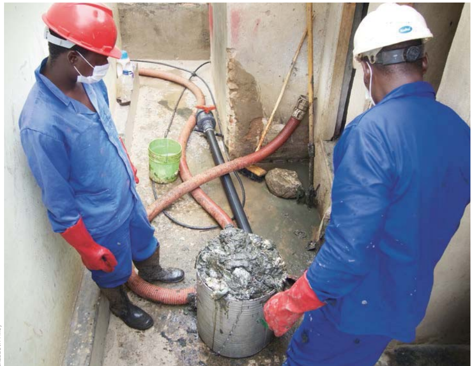
Photo 1: Sludge-soaked trash that has been fished out of a pit.
