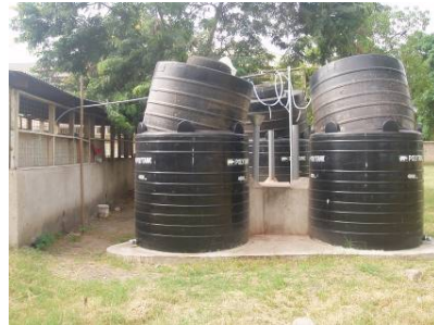
E Gas holders at their full capacity (seen tilted at the top of digester tanks), condensed water trapped where plastic pipes bent mostly, hard tube on a slight angle leading into the kitchen.
