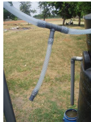
B Water trap needed to be installed near the gas holders.
