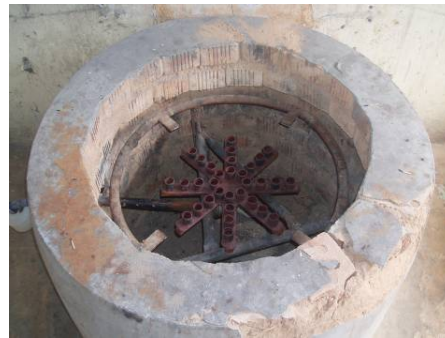
B Current gas burner at Azania
