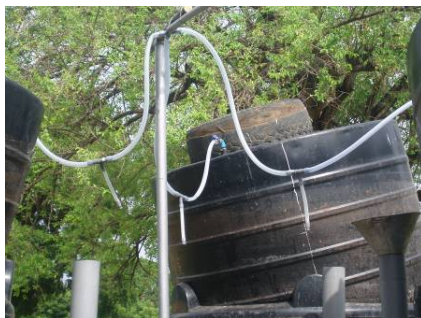
C Pipe with water traps. State of the pipes when the gas holders are full. The pipes bend so that condense water can be taken away through the water traps.
