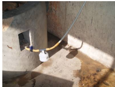
I Inlet of gas into the gas stove. Additional water trap and the gas valve placed in front of the inlet.
