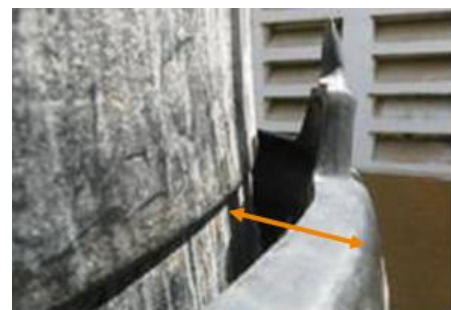
Figure 7: Biogas loss due to loose fit of the tanks
