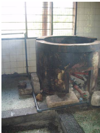
C One firewood stove at WIPHAS transformed into a biogas stove
