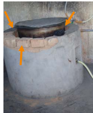
Figure 24: Biogas stove, arrows showing space for heat loss and broken bricks
