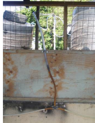
G Change of 0.75 inch pipe from outside to 0.5 inch inside the kitchen in order to increase the pressure. Two outlets to each gas stove.
