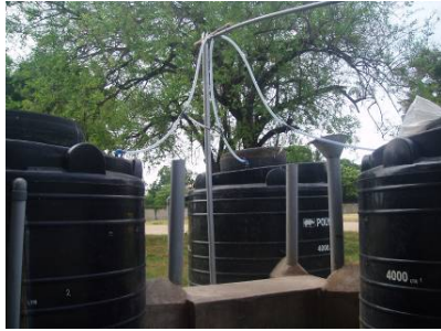
D Condition of the pipes when the gas holders are empty. The idea was that the condense water would flow back into the tanks, so that no water trap would have been needed. Accumulation of water occurred in front of the gas valve causing blockage of the outlet gas pipe.
