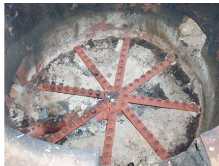
D Gas burner at WIPHAS
