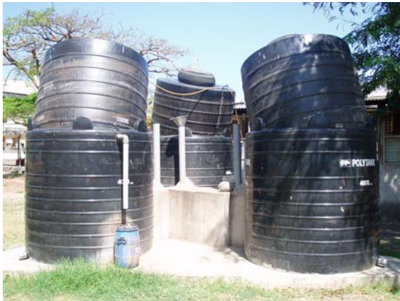
Figure 1: Three ARTI Compact Biogas Systems at Azania Secondary School
