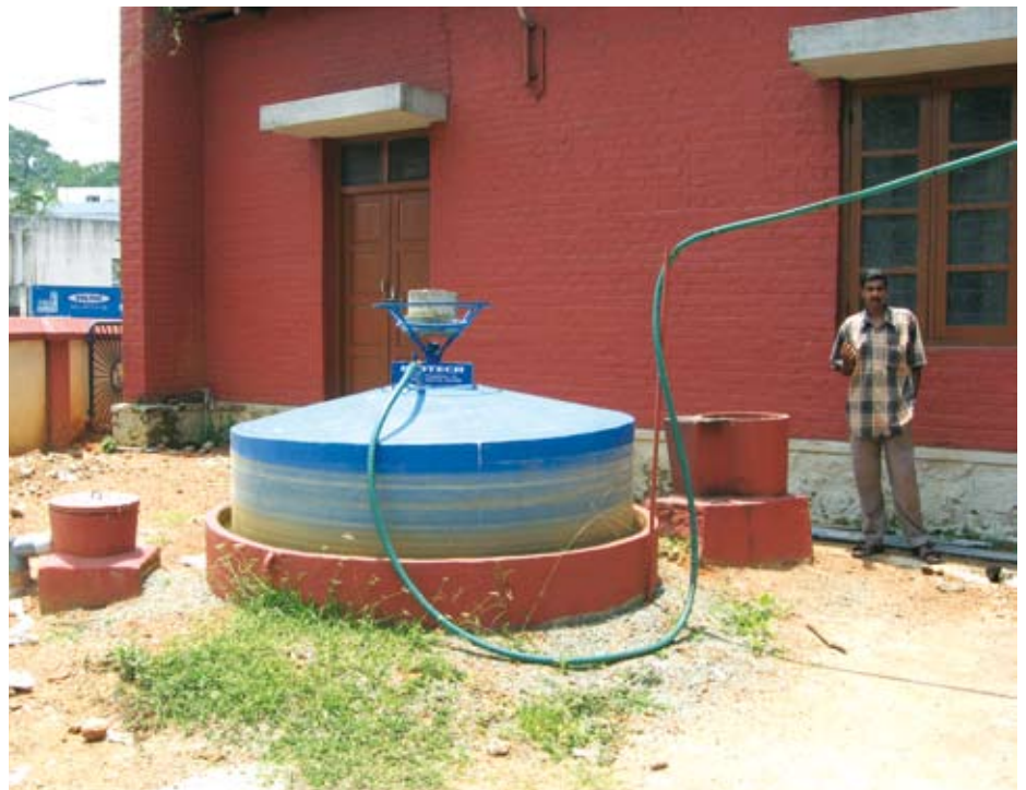
Photo 1: BIOTECH biogas plant fed with canteen waste (30 kg/d) in Trivandrum, India.
