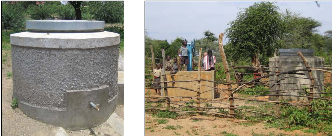
Figure 3-3: The picture on the left shows a remote community filter for treating surface water. The picture on the right shows a remote community filter that is attached to a hand pump unit for pumping groundwater.
