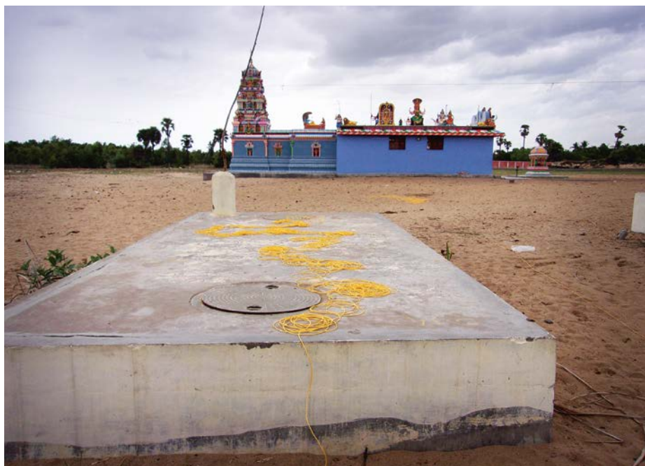
Photo 1: Primary treatment component of a community treatment plant in Tamil Nadu.
