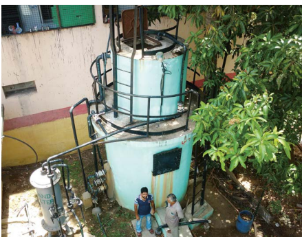
Photo 1: Basic assessment visit of a small-scale sewage treatment plant in Chennai, India.
