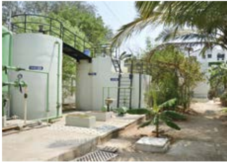
Photo 1: Small wastewater treatment plant for office buildings in Chennai, India.
