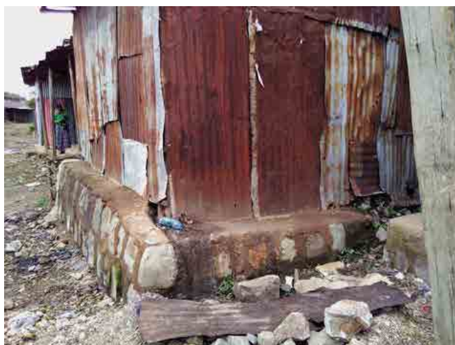
An overflowing pit latrine, Welkite. (Photo credit: Kathy Eales).
