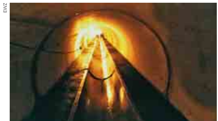
Fig. 1: A 200 m-long heat exchanger integrated in a sewage pipe.
