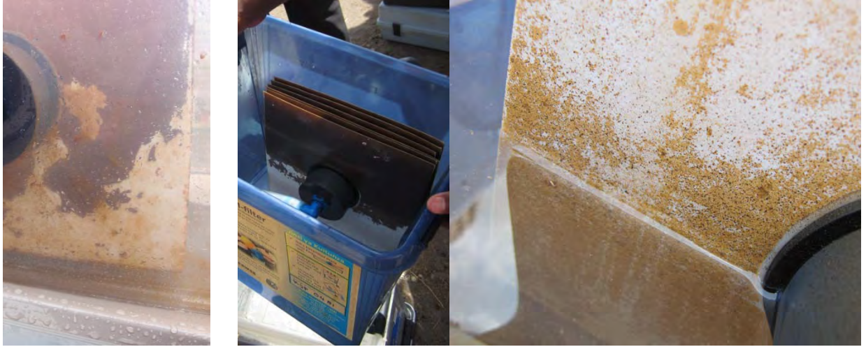
Figure 41 Pictures of the membranes showing sloughing of the biofilm after 3-6 month of operation (Photos: M.Peter, S.Derksen)
