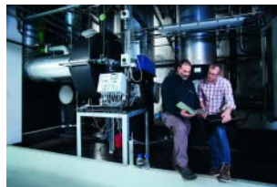
Air-stripping installation for nitrogen recovery at the Opfikon wastewater treatment plant.
