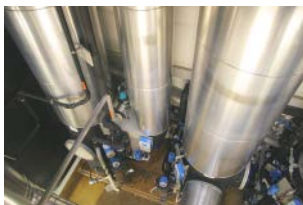
Air-stripping installation for nitrogen recovery at the Opfikon wastewater treatment plant. Photo: Eawag, Yvonne Lehnhard
